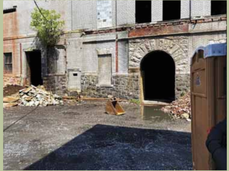
The arched main entrance and windows, which were bricked up for many years, are open once again. A metal sign for the Uhl's brewery once hung above it.
