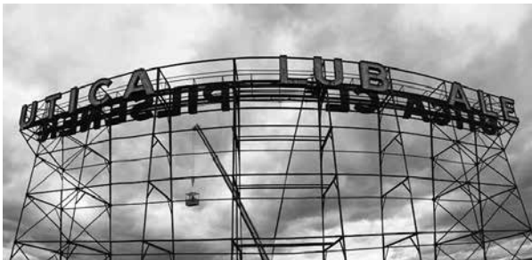
“C” you later: It was a gloomy day in April, 2016, when workers began to dismantle the sign, with the letter C coming down first. Postings on the brewery’s Facebook—clearly by breweriana collectors—suggested that the letters could be auctioned for charity.
