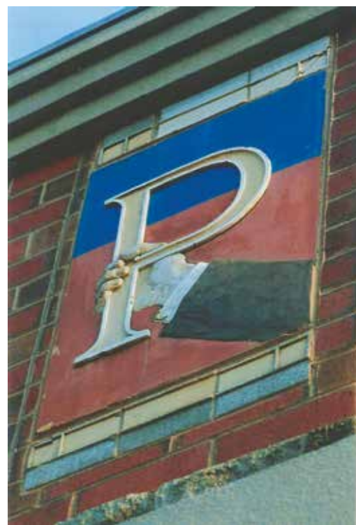
After restoration, the colors were returned to their fresh, original luster, and damage to the raised clay area was fixed (photo taken in 1997).
